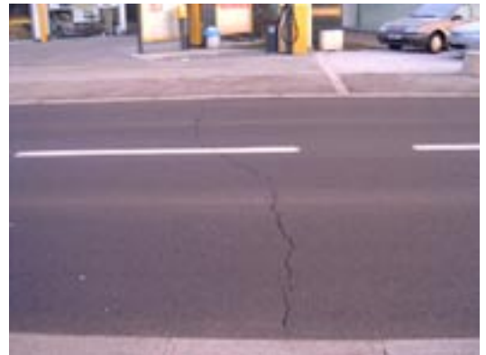
Fissure chaussée RN83 - Baume-les-Dames (Photo DDE)
